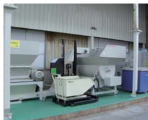
▲ Sludge solidification equipment at the KOFU Plant
